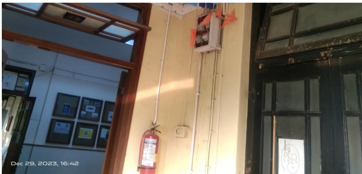
Plate 11: Fire extinguishers in the premises
