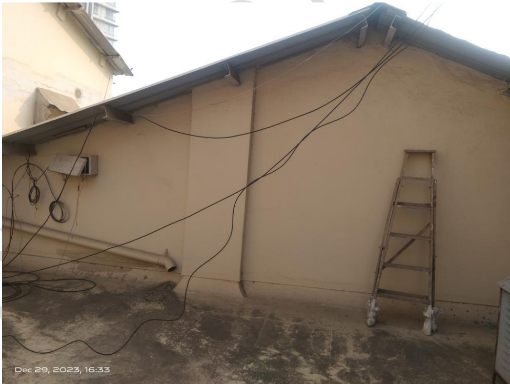
Plate 9: Exposed wiring on the clock tower area
