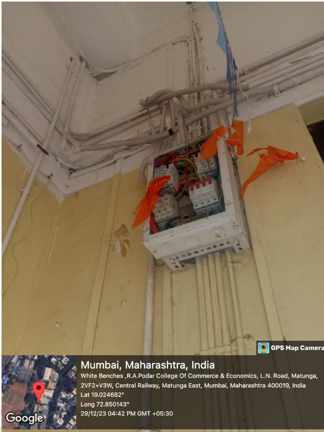
Plate 10: Exposed switchboard in the interiors of the premises
